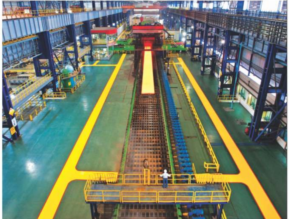
Essar Steel's 1.5 MTPA extra-wide Plate Mill at Hazira, India
